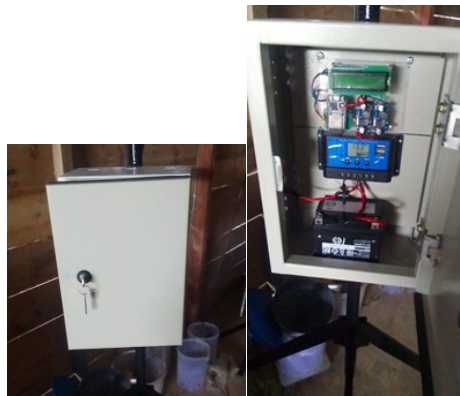
Fig. 5. Control Tool Box Panel
